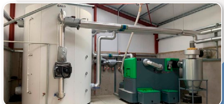
Biomass boiler 500kW
